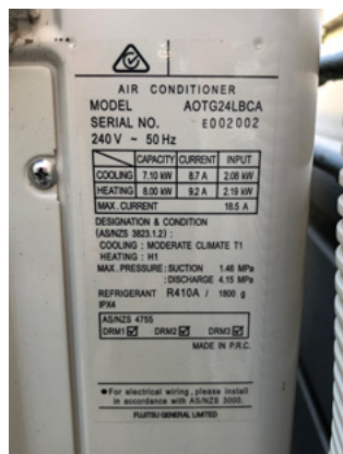
Figure 9.6 Example of a nameplate on an outdoor unit
