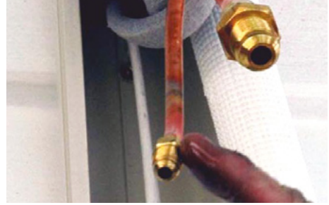
Figure 6.21 Apply oil to the back of the flared pipe and the flare joint
